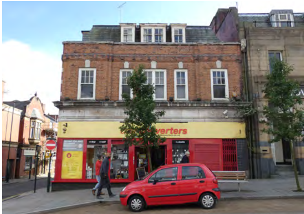
Plate 5.32 Impact of poor quality retail frontage, roller shutters and signage on quality of building above at 22-24 Yorkshire Street
