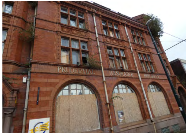
Plate 8.3 The Prudential Building, vacant and in a deteriorating condition
