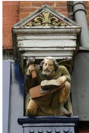
Plate 9.10 Carved capital and corbel brackets to 19 th century retail frontage on Henshaw Street
